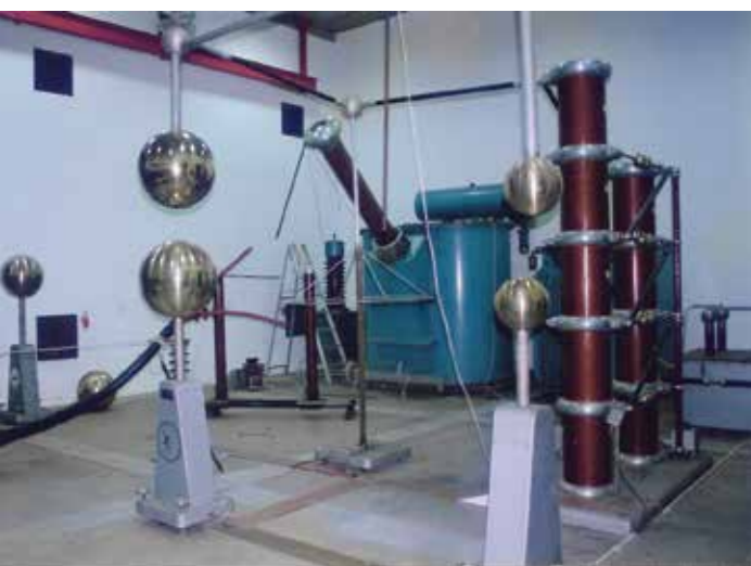
The High Voltage Laboratory sponsored by a consortium of donors that includes African Cables, Eskom, Spoornet and Transwerk
