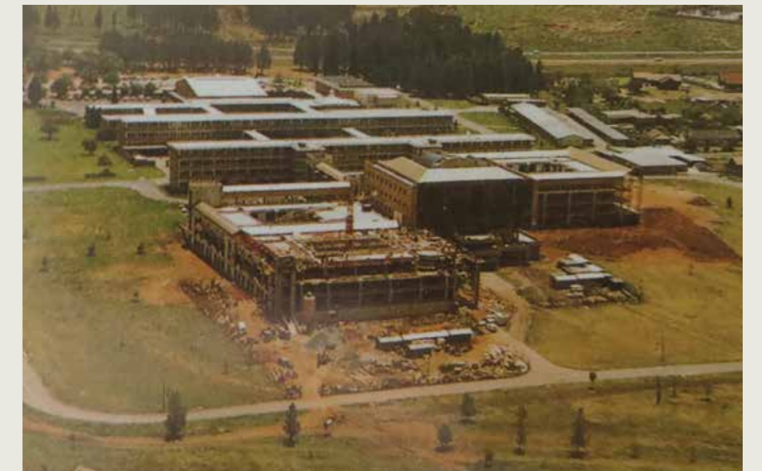
Construction begins on the new building for the Department of Human Sciences
