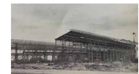
Extensions to Iscor's steel melting plant and cold mill at Vanderbijlpark Works under construction by Dorman Long
